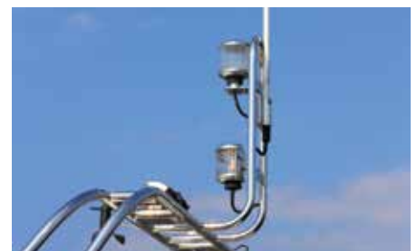
VHF antenna with duplex antenna splitter
